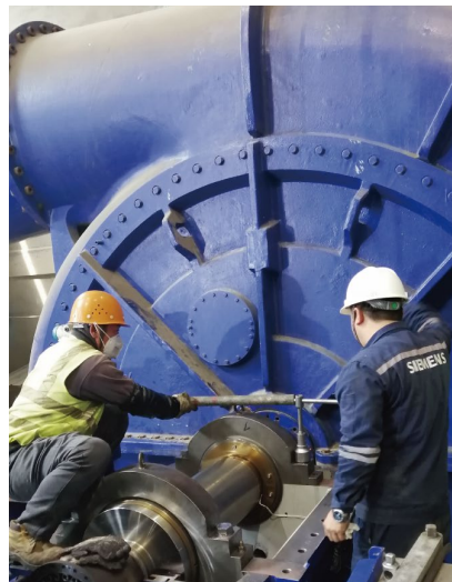
3k风机检查保养 3k Fan check and maintenance
